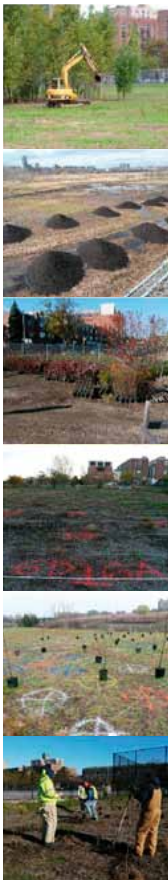
FIG. 13. Sequence of activities to implement the biodiversity study in New York, including site preparation, soil amendments, plant procurement, marking the plots, and planting (Photos: Alex Felson).
