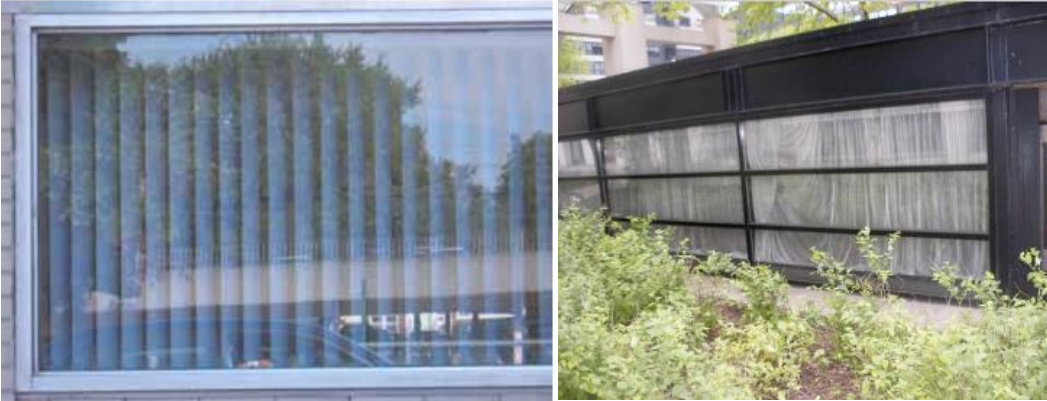
Partially open blinds (left) and curtains (right) are examples of interior elements that can reduce reflections, thereby mitigating bird strikes. Image credits: Christine Sheppard (left) and Chicago Bird Collision Monitors (right)
