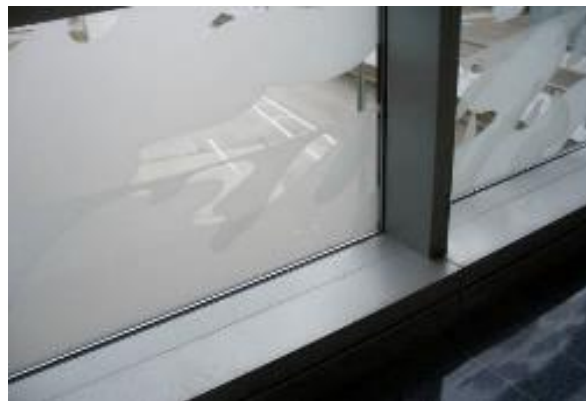
The use of frosted glass can help to mitigate bird strikes. Image credit: Chicago Bird Collision Monitors
