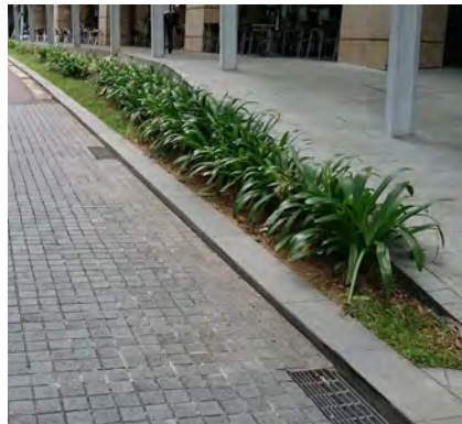
Remnant grass patches are unproductive for grasscutting. Narrow strips should be fully replaced by groundcovers.
