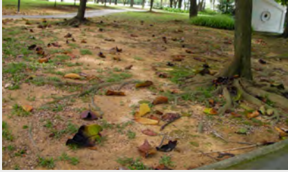
Exposed and shallow roots have caused uneven surfaces. It restricts continuous machine mowing and a knapsack cutter has to be used.
