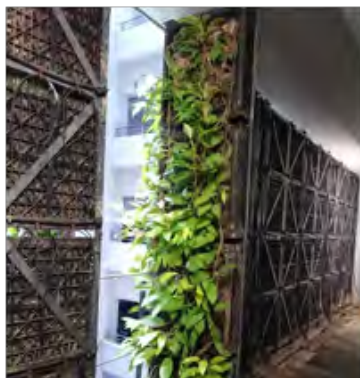
‘Open-able’ vertical greenwall panels and service walkway with back access at the National University Hospital
