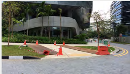
The grass is being protected to reduce the impact of heavy vehicular path and should be properly reinstated after completion of work.
