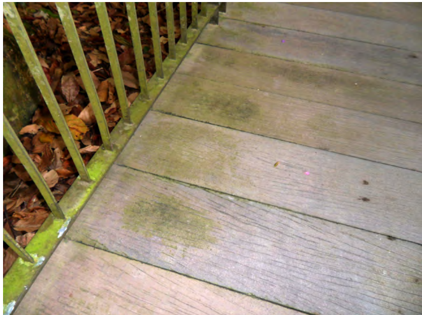
Algae on timber deck can be a slipping hazard
