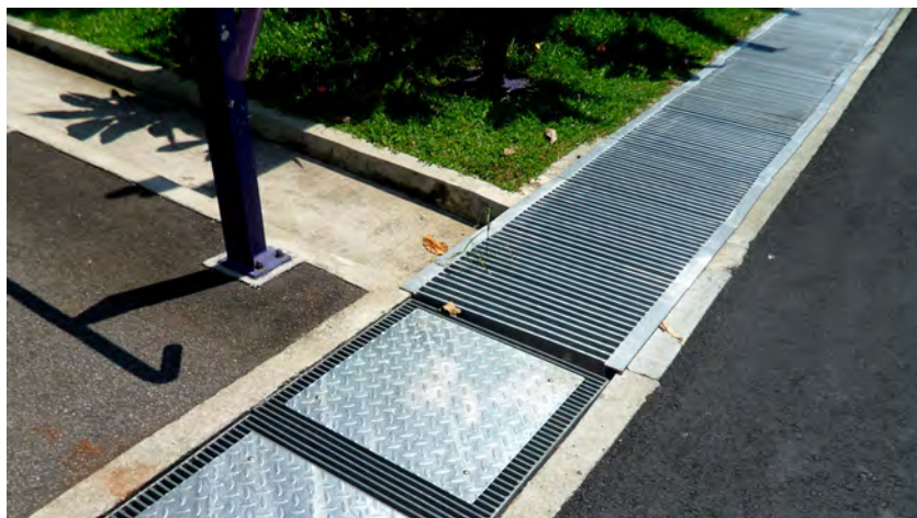
Galvanised steel plates and gratings over drains
