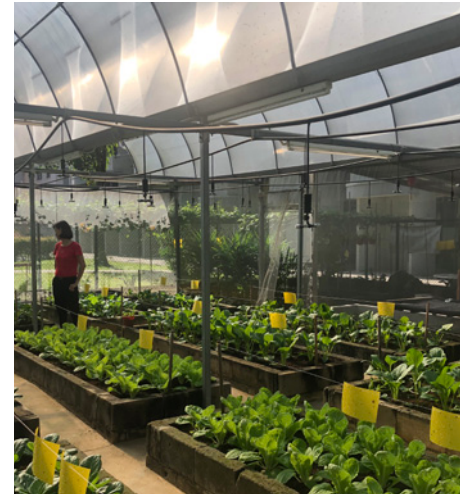
Overhead type of sprinkler system at Teck Ghee Jubilee RN
