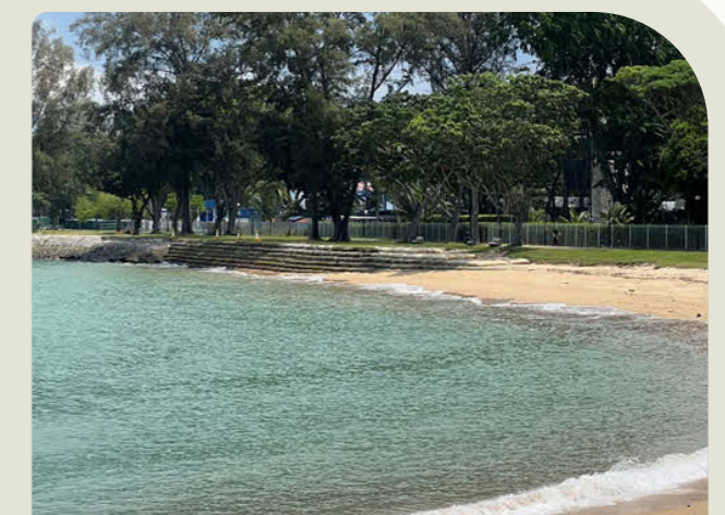
Completed NEWSand geobags installation along a segment of the coastline at East Coast Park.
